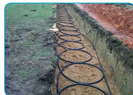
Ground Source: Ground Loop
